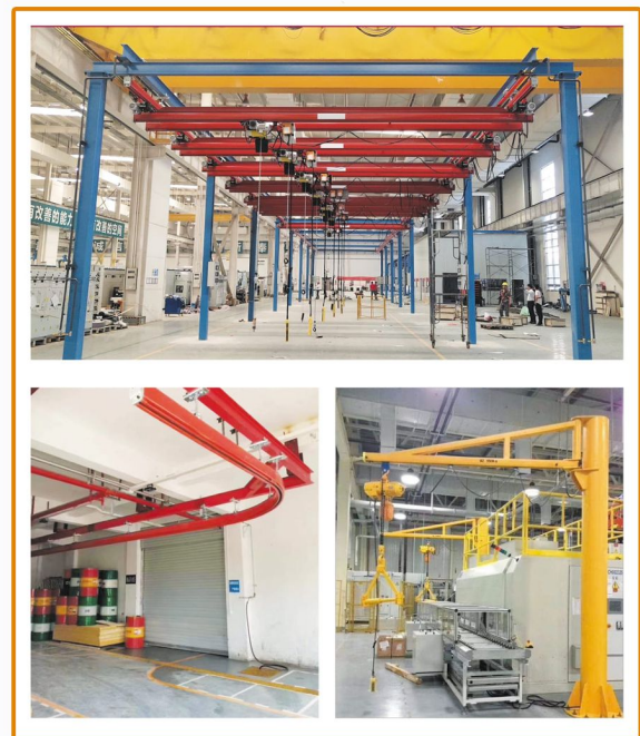
LIGHT CAPACITY CRANE
